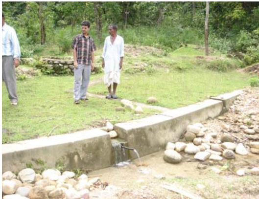
(Intake protection Jamuna WSSP BVI Sindhuli SO IRDS)
