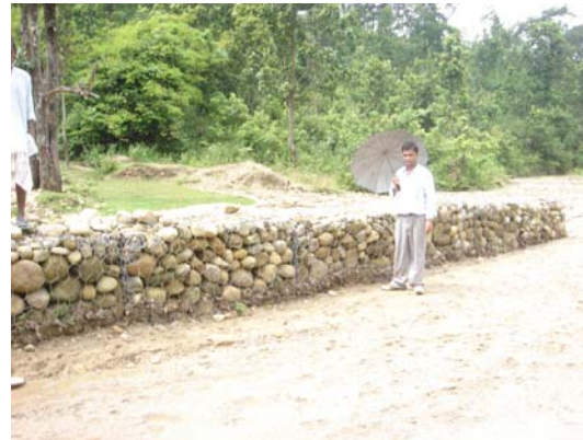
Pipe line protection Khorkhola WSSP BVI Sindhuli SO IRDS
